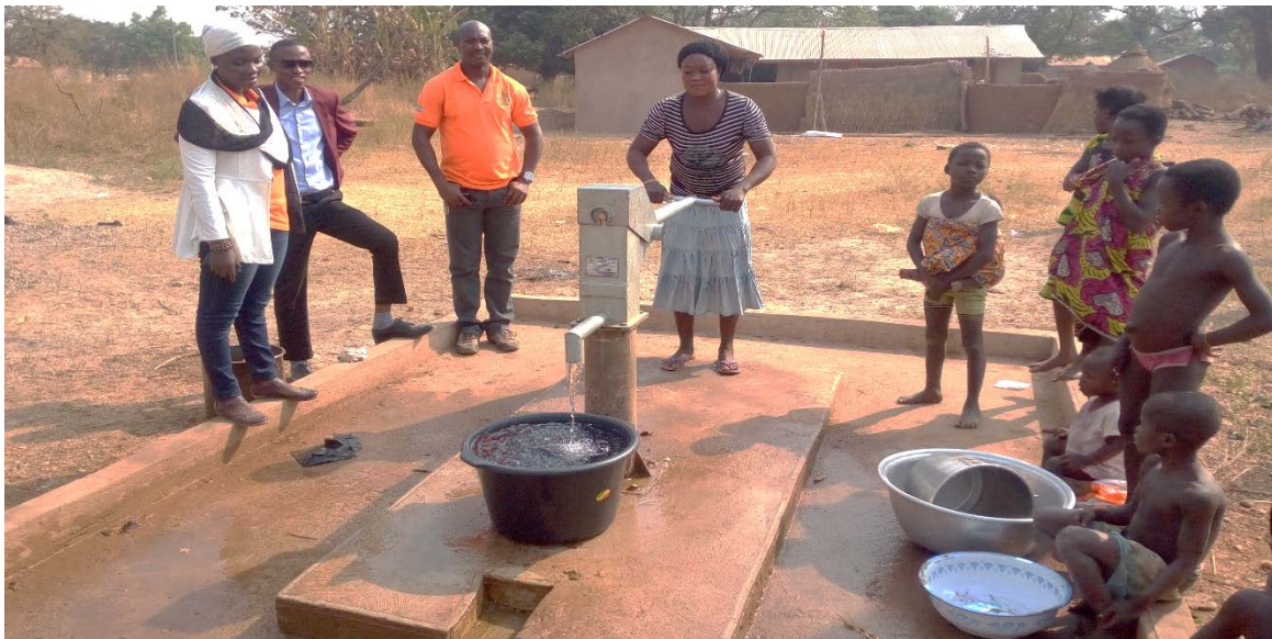
Figure 10 Regional and District monitoring team observes functionality of borehole after repairs (Gbingbaliga community)
