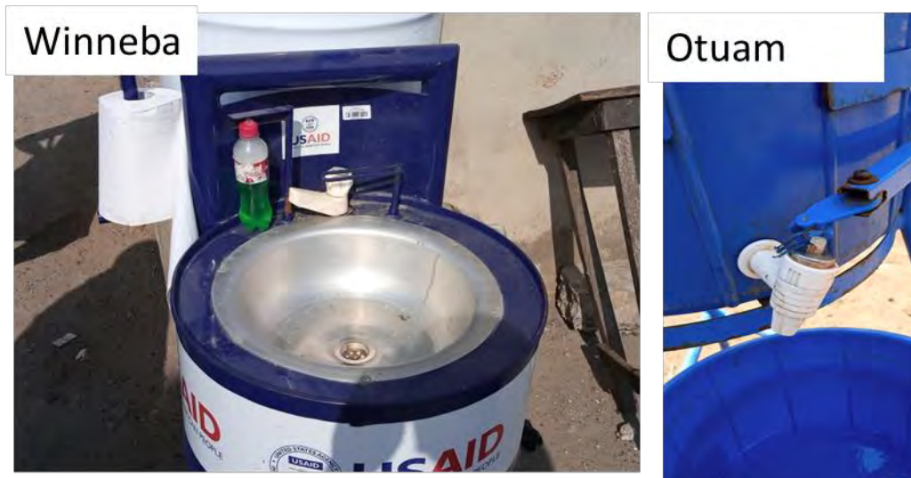
Figure 8 Broken taps replaced with improvised taps
