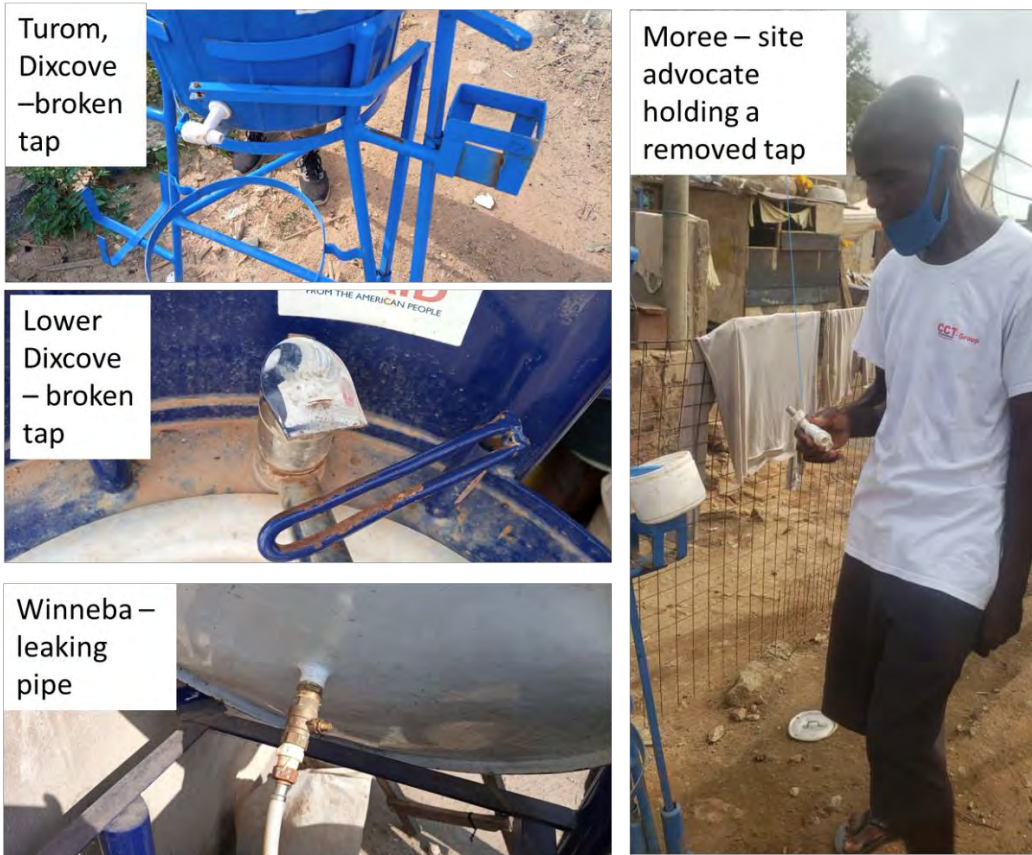
Figure 6 A sample of handwashing stations with broken taps and leaking pipe
