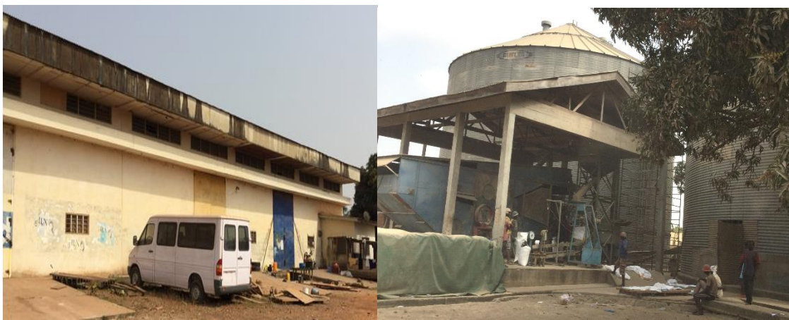
Plate 3: Dilapidated warehouses at Sunyani
