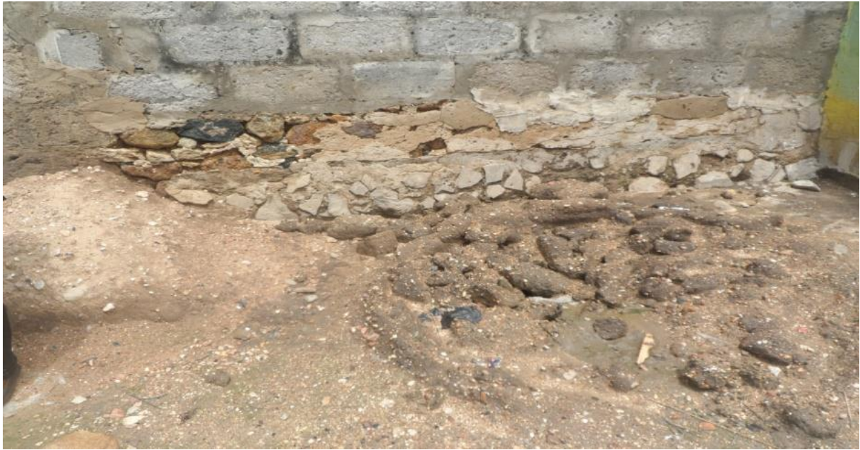
Plate 8 Bad Oven (totally collapsed in Winneba community)
