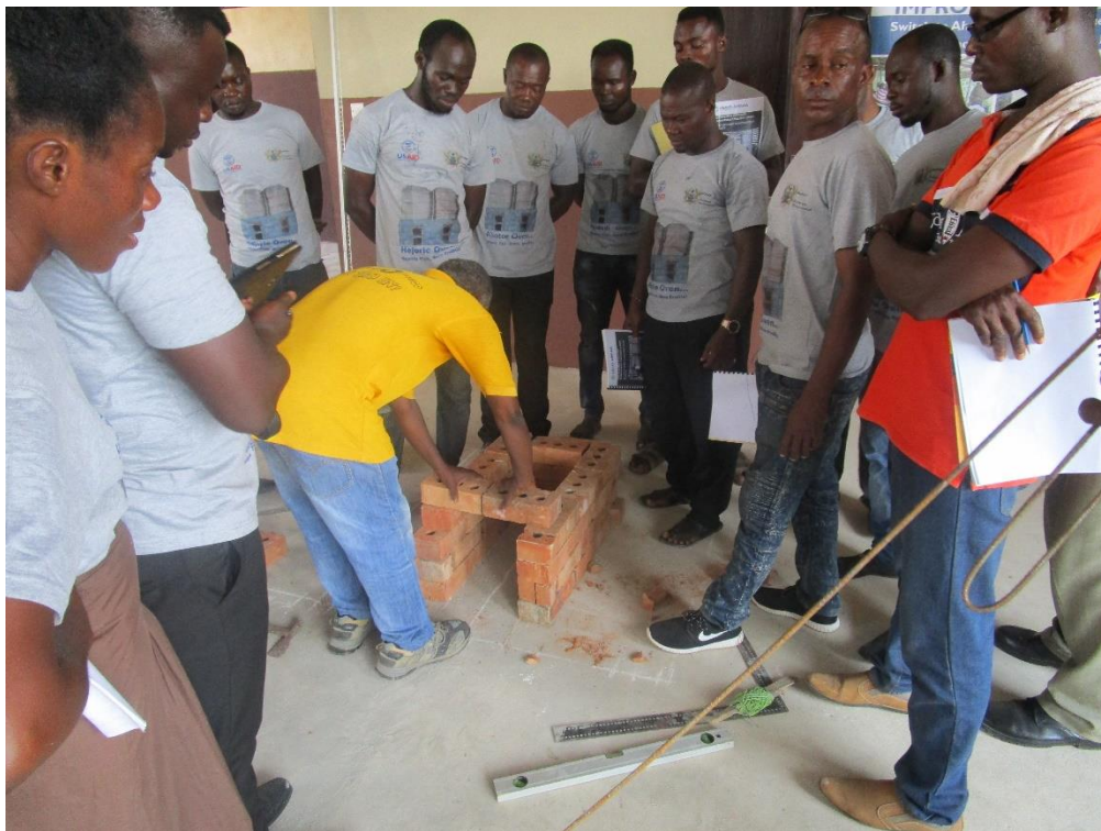
Figure 3. Training of artisans at Elmina on how to construct the Ahotor oven
