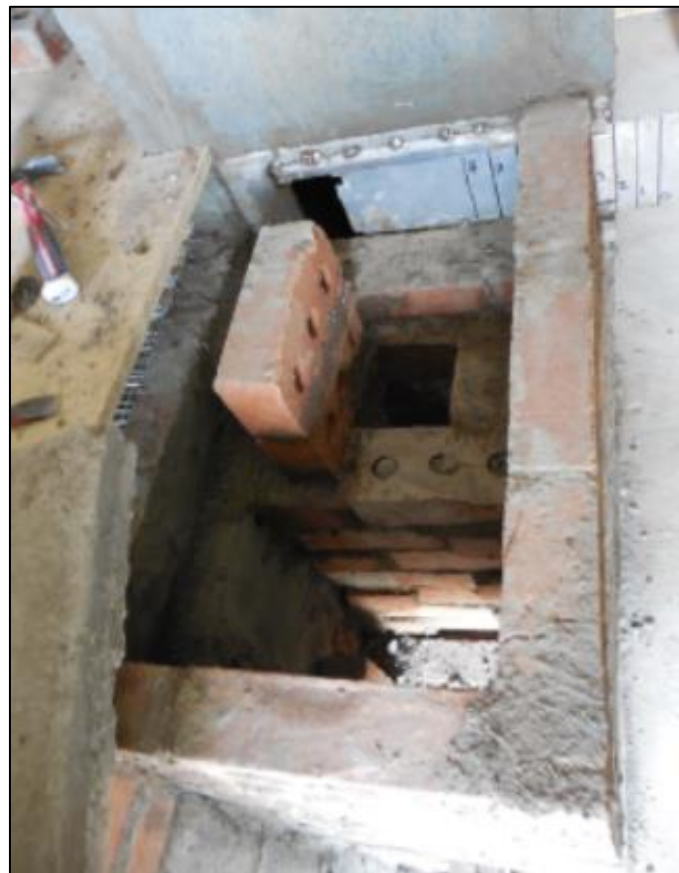
Figure 14 Top of the flame tunnel
