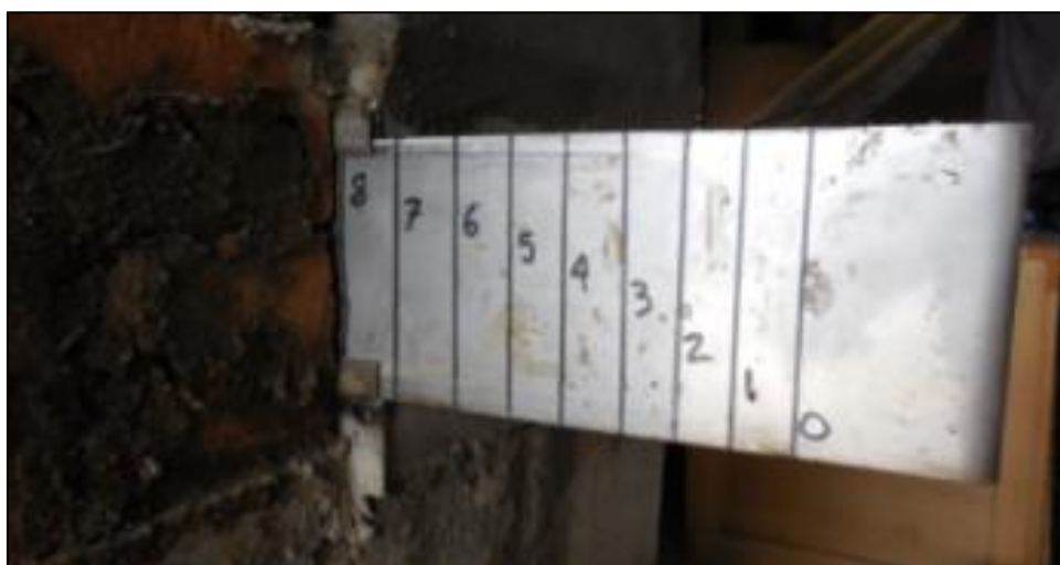
Figure 11 By setting the opening, the level of heating and thus the chimney draft can be regulated
