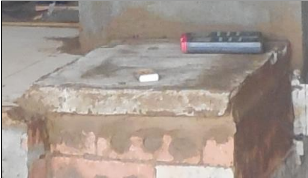
Figure 15 Heat resistance cover at the top of the fire chamber
