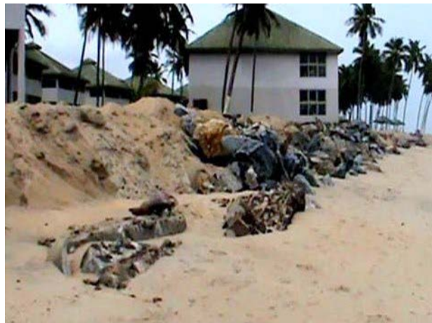
Figure 10: Coastal infrastructure under threat in the Central Region
