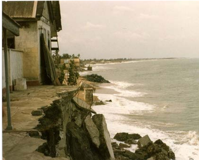
Figure 2: Collapsing coastal structures in the Volta Region
