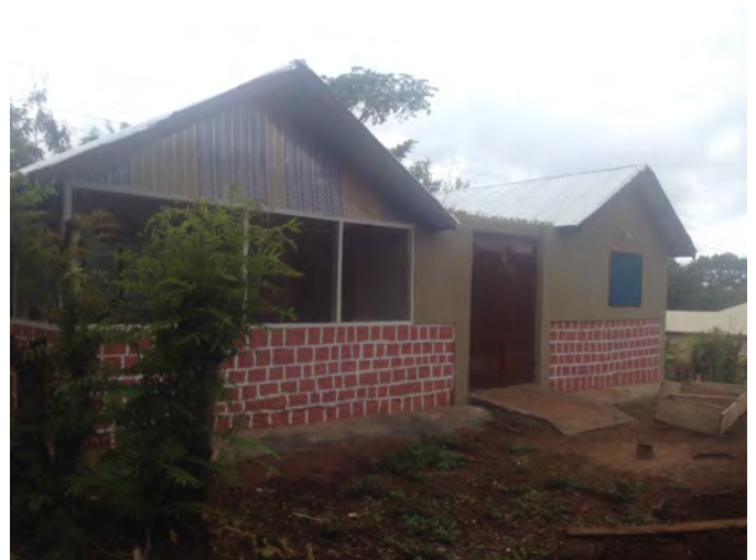
The Bodaa Community Cashew Apple Processing Facility will be used to provide income to community members while at the same time promoting and providing improved nutrition.
