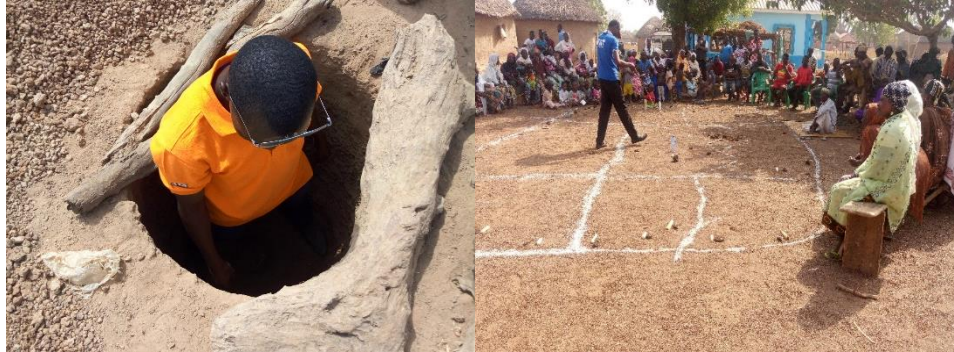
Photo 13 (L) Latrine construction in progress and (R) community triggering in Nafarun, Tolon District
