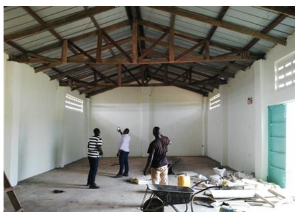
Nestle Procurement Manager inspecting the newly constructed warehouse of Kharma Farms in Karaga, Northern Region
