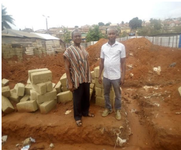
Chairman and secretary of the Techiman Maize traders’ association at the construction site of the on-going washroom facility construction at Techiman
