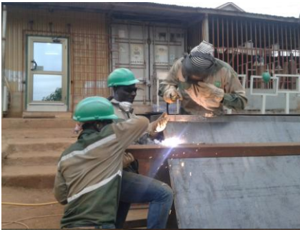
Photo: Wayoe Eng. welding staff utilize PPE best practices as realized during SCD Trainings in Takoradi
