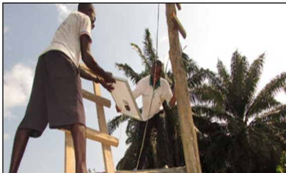
Figure 27 Solar Installation at Eshiem
