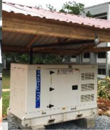
Installed 65 kVA generator
